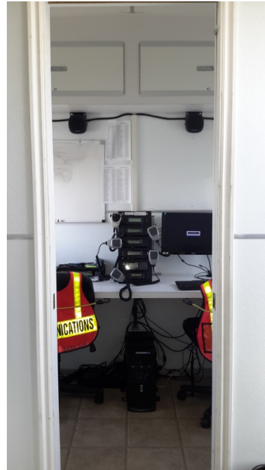
Communications Room of Search & Rescue Command Post Trailer
